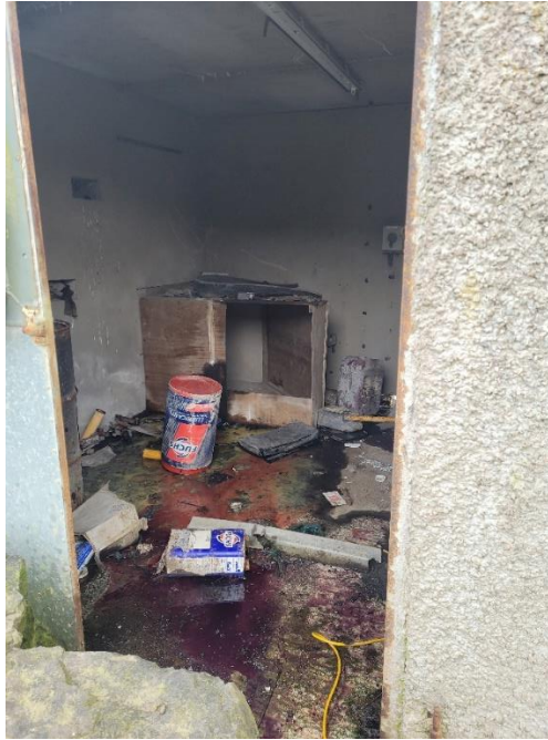
Figure 4.3 Derelict Building Containing Potential Chemical Spills
