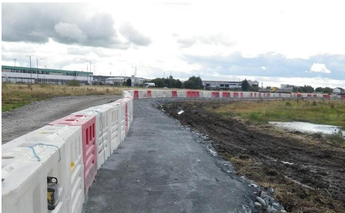
Figure 15 – Example pedestrian / vehicle segregation on haul road
