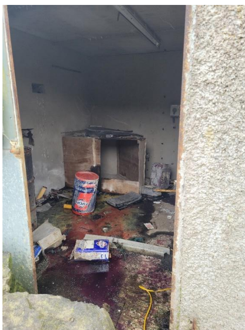
Figure 8.3 Derelict Building Containing Potential Chemical Spills
